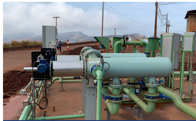
Pre-Filtration for Water Treatment
