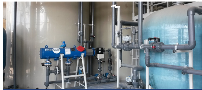
Industrial Process Water Installation
