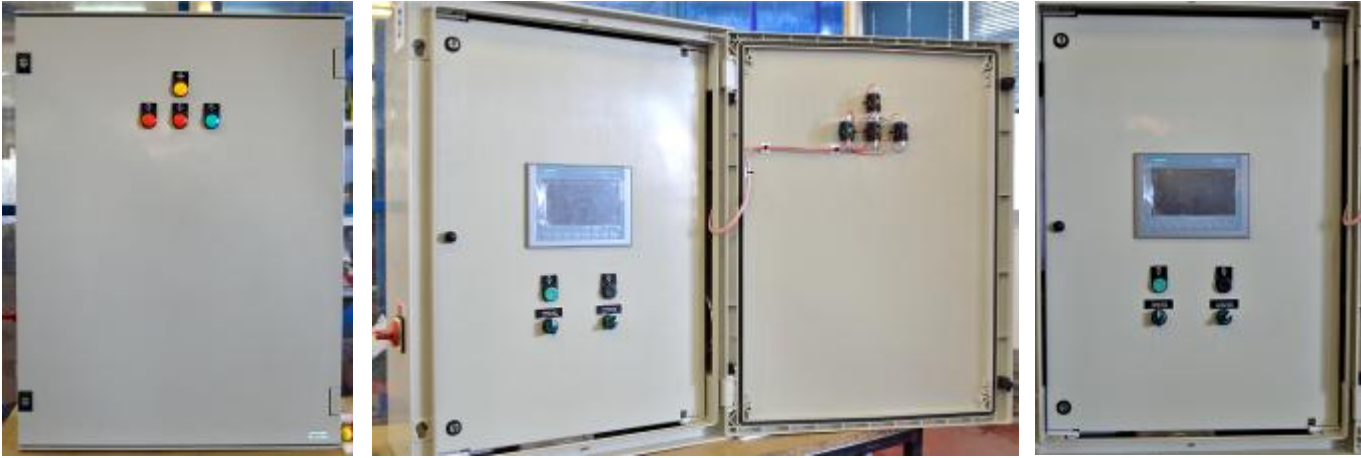
The Sub-Master Control Panel
